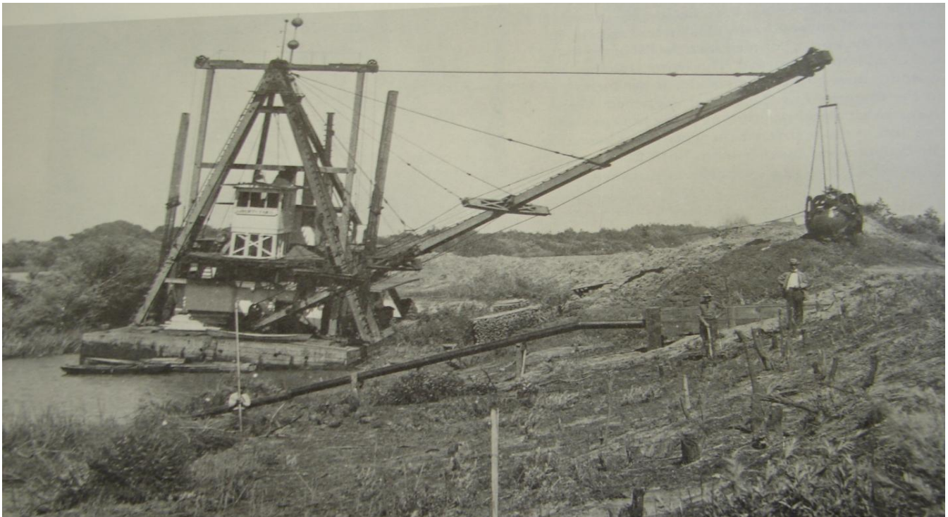
Figure 1. Construction of a Levee by Clamshell Dredging in California around 1910 (from Sacramento Archives & Museum Collection Center)
